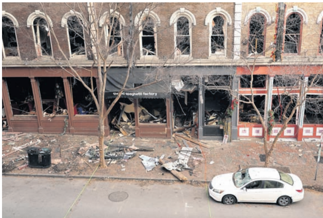
In this Dec. 29, 2020 file photo, debris remains on the sidewalk in front of buildings damaged in a Christmas Day explosion in Nashville, Tenn.
